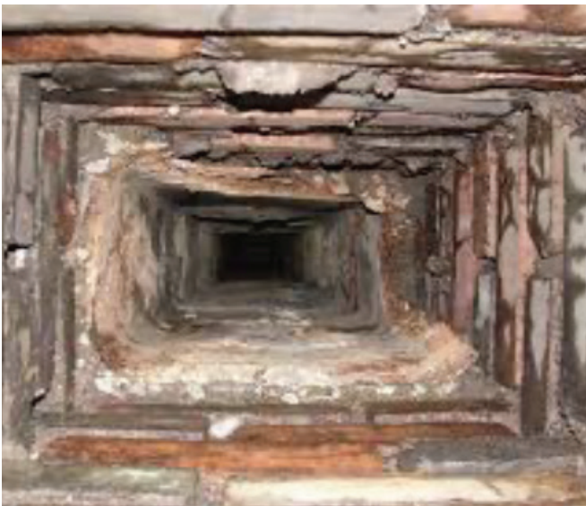
Figure 4: Inside of an old brick chimney unsuitable for modern appliances.
